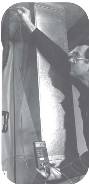
FIGURE 48 TEMPERATURE RISE MEASUREMENT
