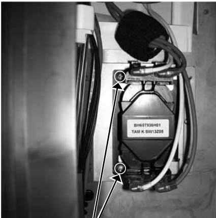
Screws of the reactor
